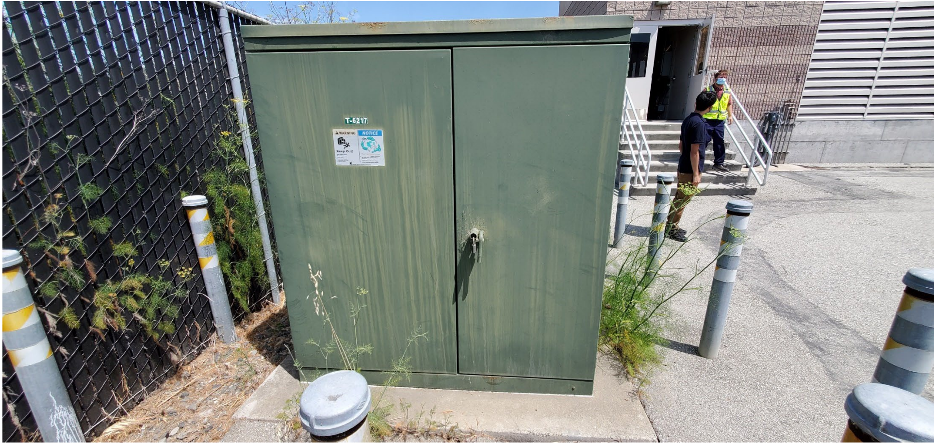
A9. Electrical box in the Pump Station 4 area.
