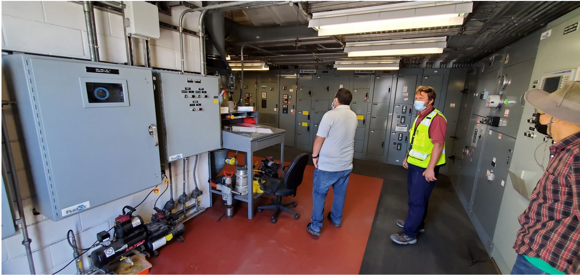
A6. Example of electrical systems inside a building in the WQCP area.
