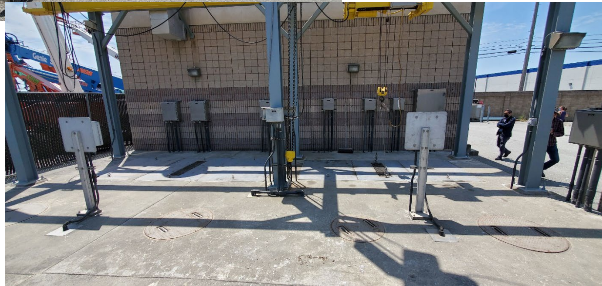
A8. Equipment at Pump Station 4.
